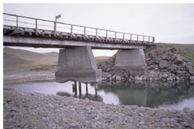
Erosion effects on bridge pier positioned in the streambed
